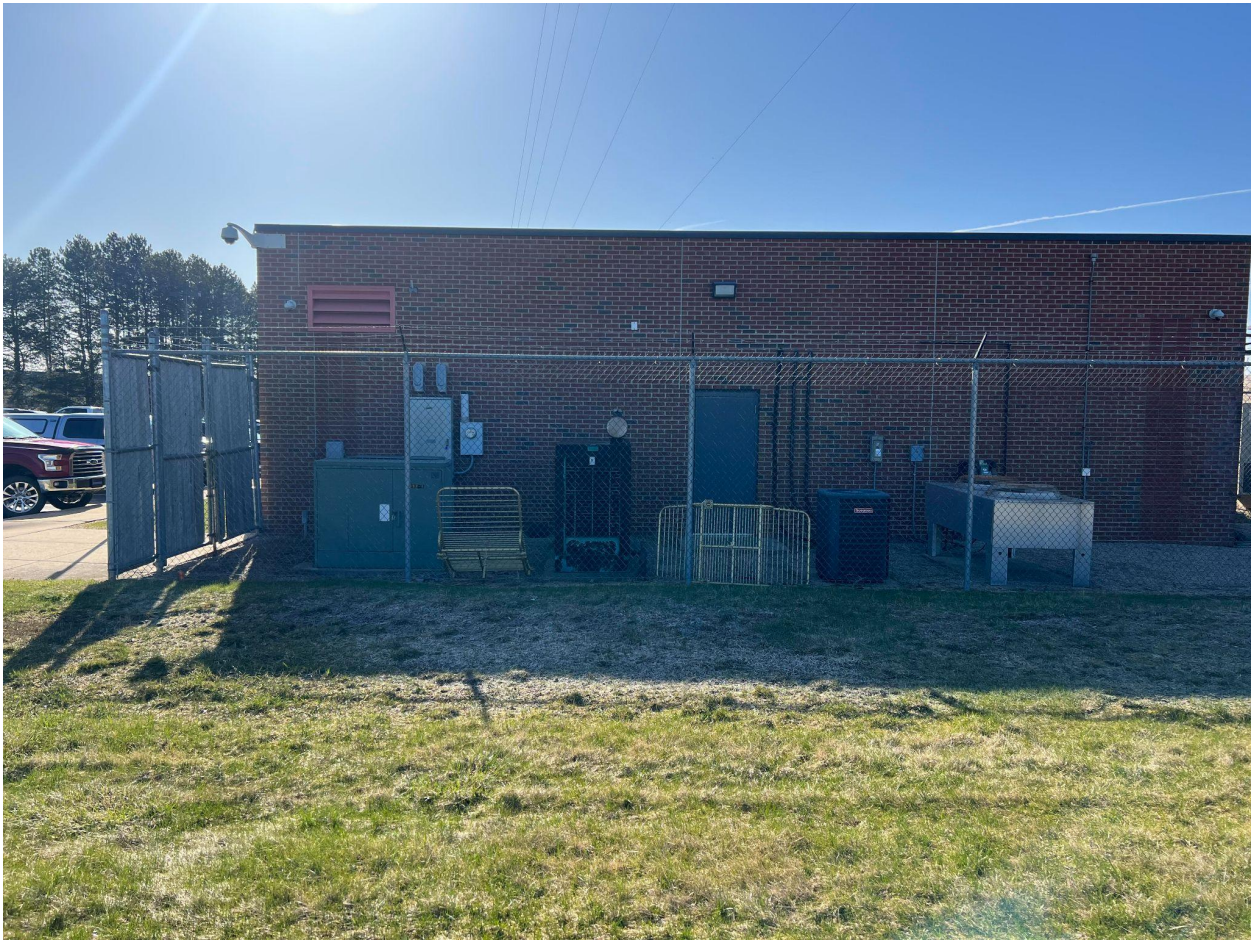
Exterior generator photo
